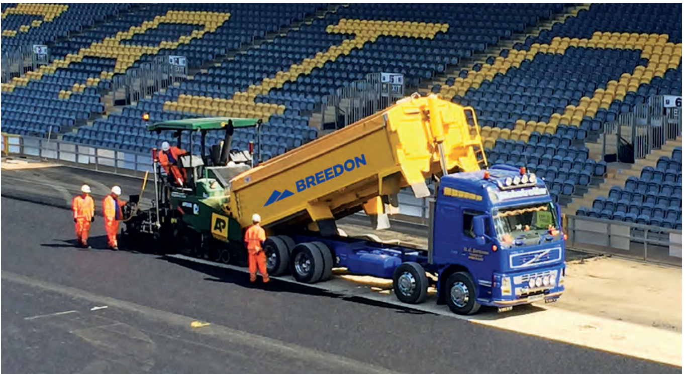
The Breedon Southern Contracting team lay a new artificial pitch to allow Worcester Warriors rugby club to stage concerts and other commercial ventures.
